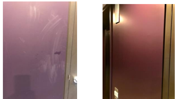
Left: This door shows typical marring. Right: Same door, repainted with Porter's Aqua Satin, and back in use.
